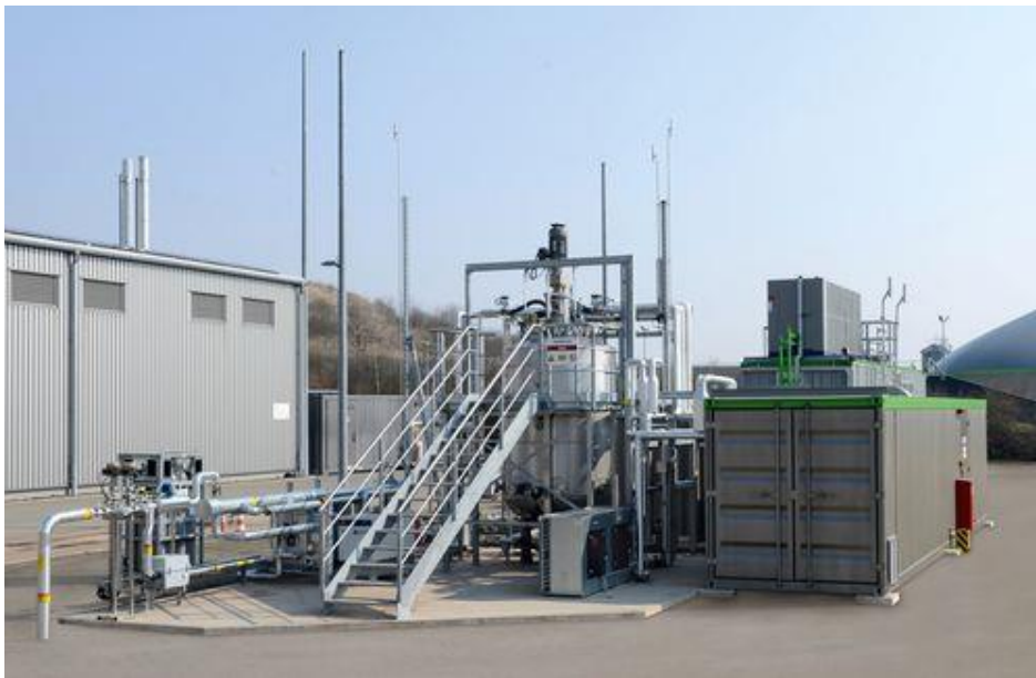
BioPower2Gas pilot plant in Allendorf
