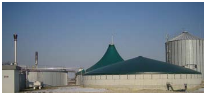
Photo 14 : General view of a 1 MW e crop co-digestion plant using two parallel digesters (left background) and a covered final digestate storage tank (centre foreground). Gas storage is integrated in digester 2 (background) and in the final storage tank (foreground), further storage capacity is provided in a dry gas storage tank (background right).
