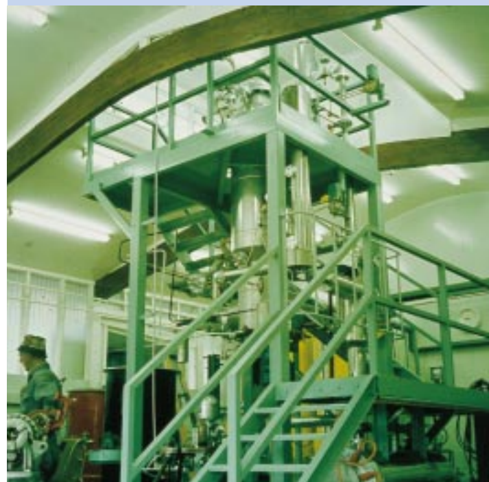
Left: Ethanol pilot plant in Rotorua, New Zealand.
