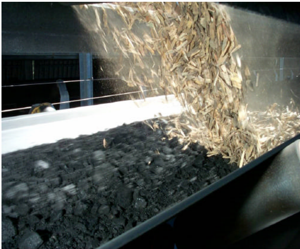
Figure 10 Wood chips are metered directly on a coal conveyor before the mills at Wallerawang Power Station, Australia (Courtesy of Delta Electricity, Australia).
