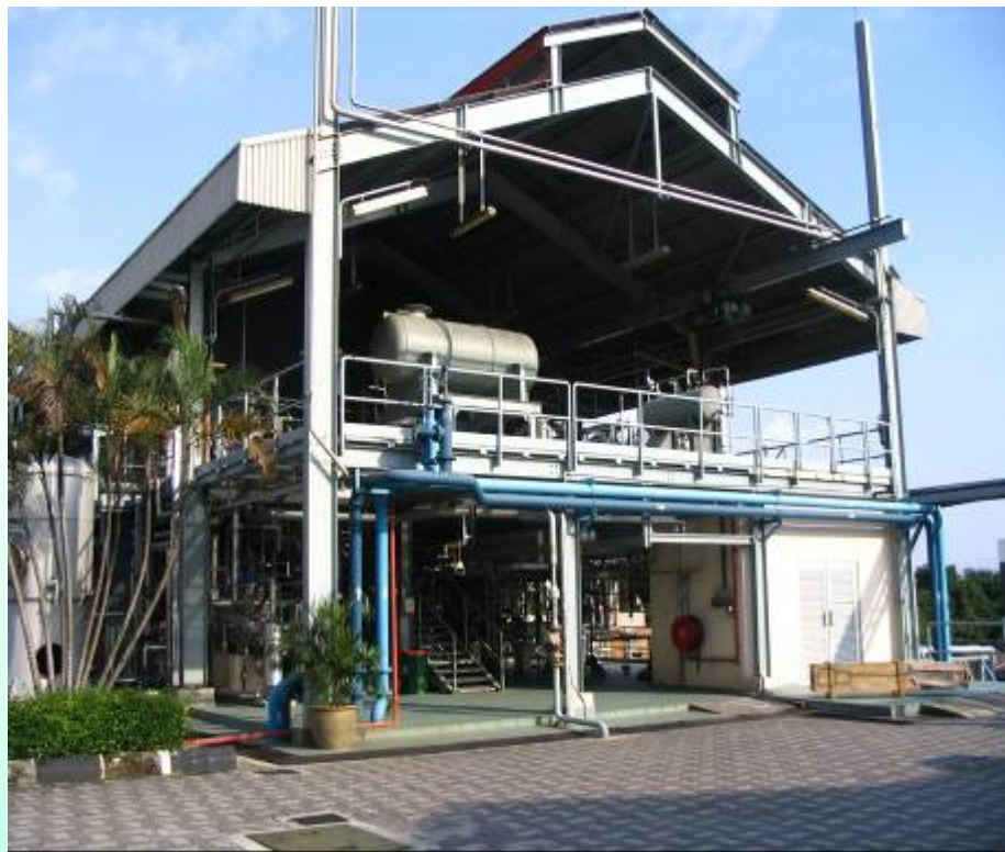
MPOB Palm Biodiesel Pilot Plant
