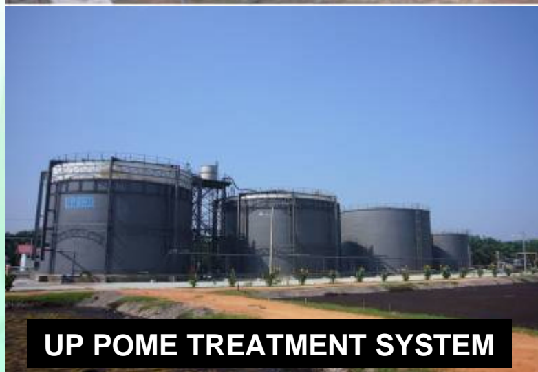
PONDS & TANK DIGESTER
