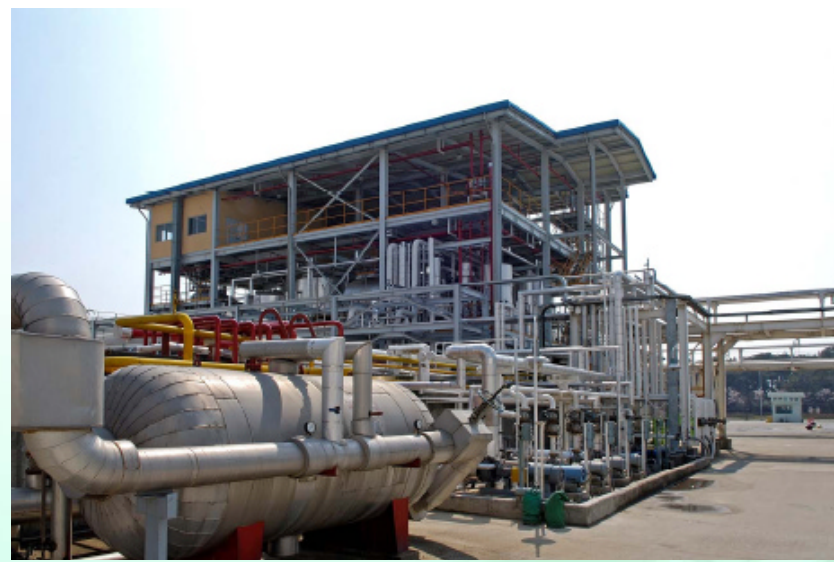
Front view of Biodiesel Plant
