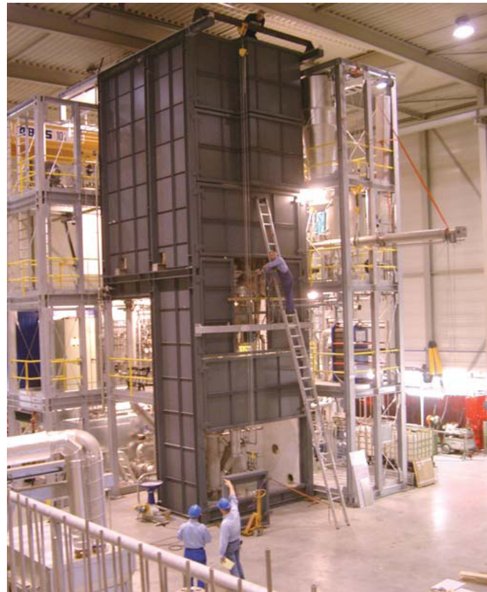
BTG 50 t/d rotating cone fast pyrolysis plant, Malaysia
