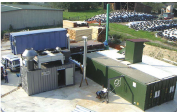
PyTec 50 t/d ablative pyrolysis plant, Germany
