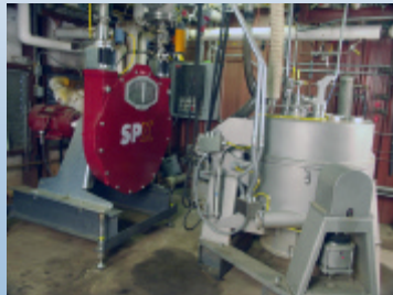
Hose Pump and Centrifuge
