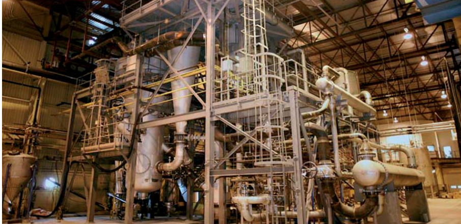
Pyrolytic liquid platform biorefinery for polymers, synthetic fuels, food, power and heat from lignocellulosic residues. Courtesy Ensyn, Canada; and Task 42.
