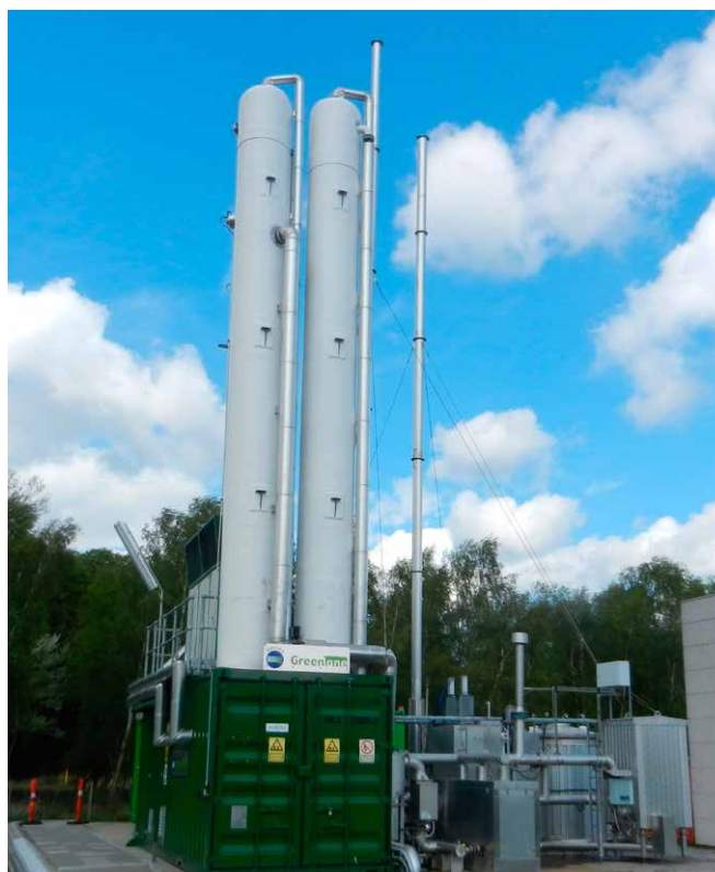
Figure 3: The upgrading plant. Source: DONG Energy.
