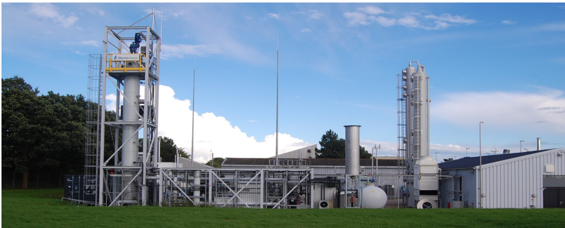
©Electrochaea GmbH, BioCat Pilot Plant near Copenhagen, DK
