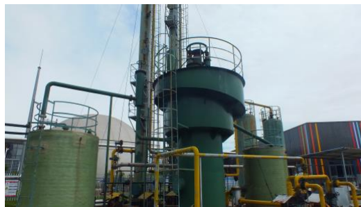
(B) Biogas desulfuration unit
