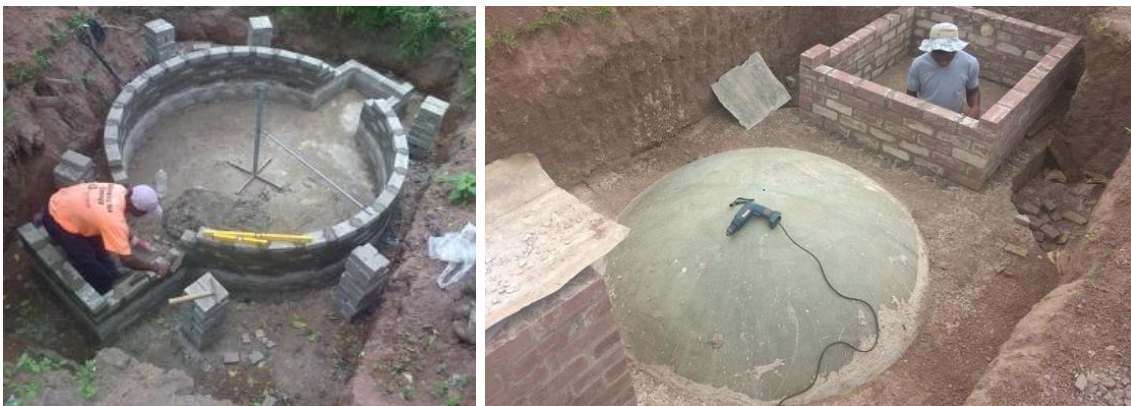
Figures 3a and 3b: 3a (top) - Plan and section of the biodigesters installed at Ndwedwe; 3b (bottom) - Photos during the installation of the household digesters. Design and photos courtesy of Khanyisa Projects and SANEDI (Khanyisa Projects, 2014)
