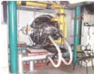
Figure 1: Co-combustion of bio-oil produced by BTG Biomass Technology Group in Electrabel's 350 MWe gas-fired power station in Harculo, The Netherlands. Photograph of the burner front side showing the pressurized bio-oil lines including the atomization pressure indicators. Reproduction of the photographs is subject to permission by Electrabel and BTG.
