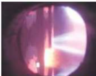
Figure 2: Co-combustion of bio-oil produced by BTG Biomass Technology Group in Electrabel's 350 MWe gas-fired power station in Harculo, The Netherlands. Photograph of the boiler room side of the bio-oil burner and its (orange) flame. Eight other burners in the boilers house (55 MWh each) were fired on natural gas (blue flame). Reproduction of the photographs is subject to permission by Electrabel and BTG.
