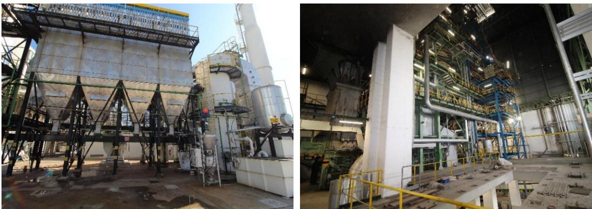
Figure 2 - On the left: the thermal area with the furnace for the combustion of SRF and the boiler for steam production; on the right: part of the flue gas treatment line.
