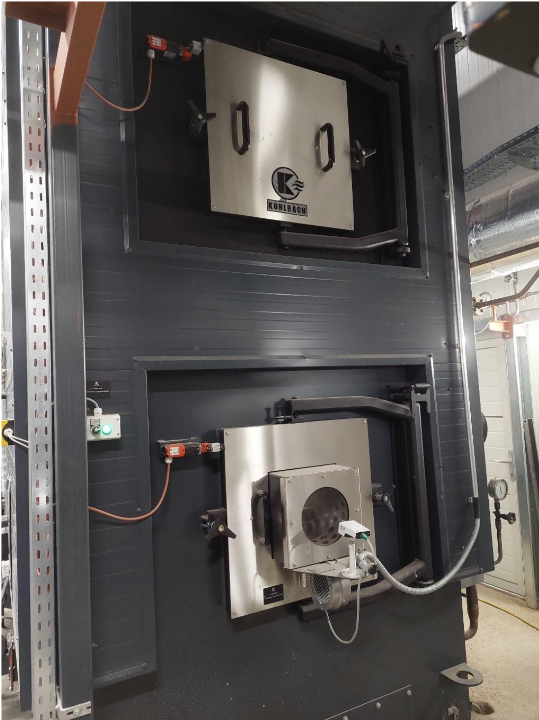
Figure 6: Furnace of the company Kohlbach (Source: BC Regionalwärme Group)
