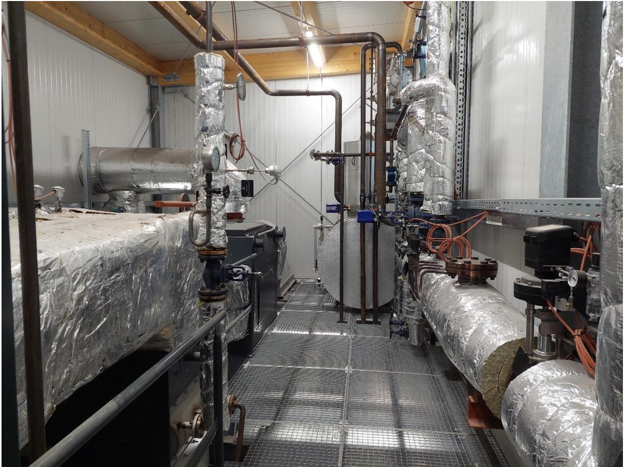
Figure 7: Economiser (front left), multicyclone (rear left), feedwater tank (rear right) and steam distributor (front right) (Source: BC Regionalwärme Group)
