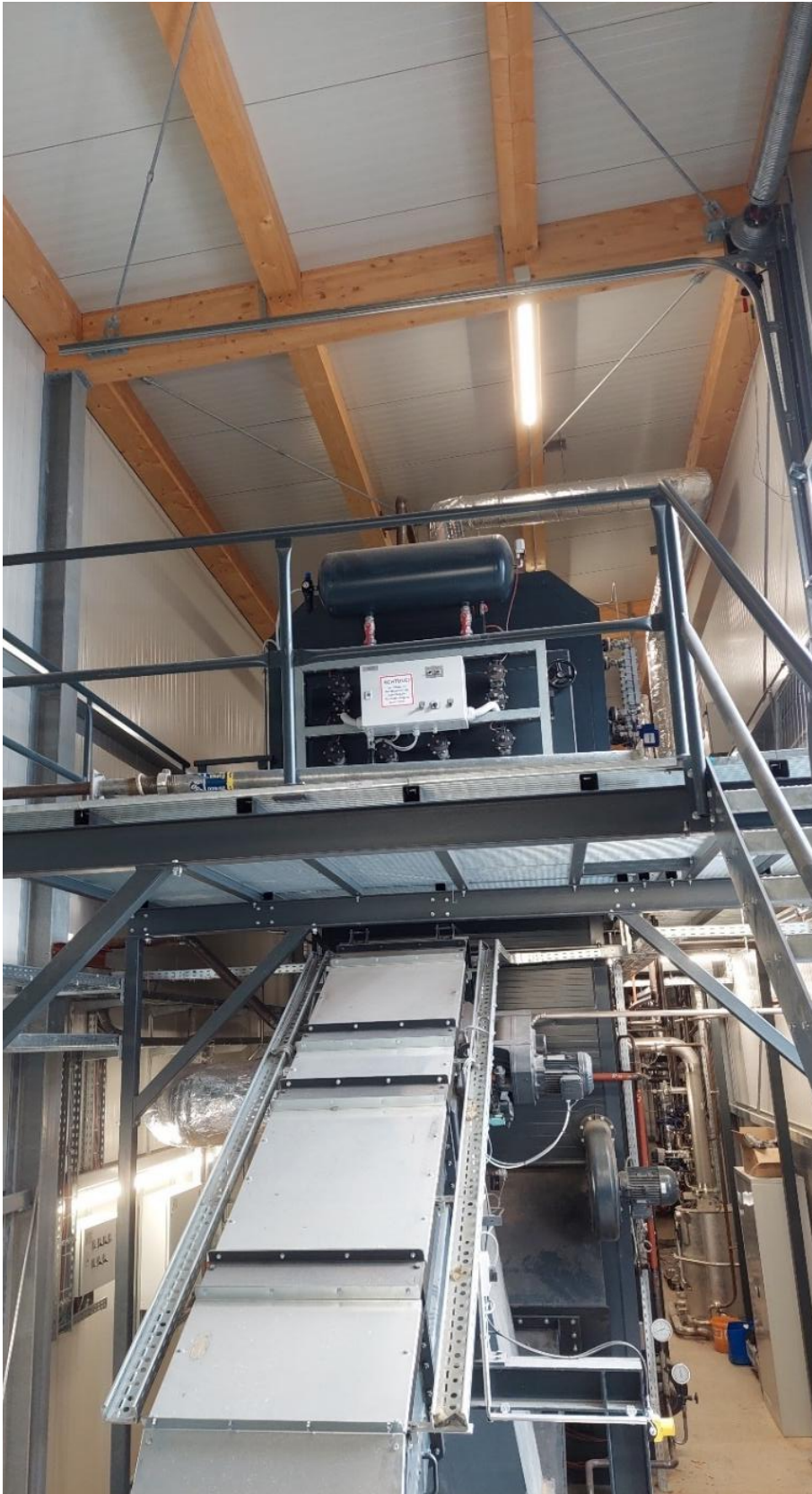
Figure 5: Furnace and steam boiler with chain conveyor (Source: BC Regionalwärme Group)
