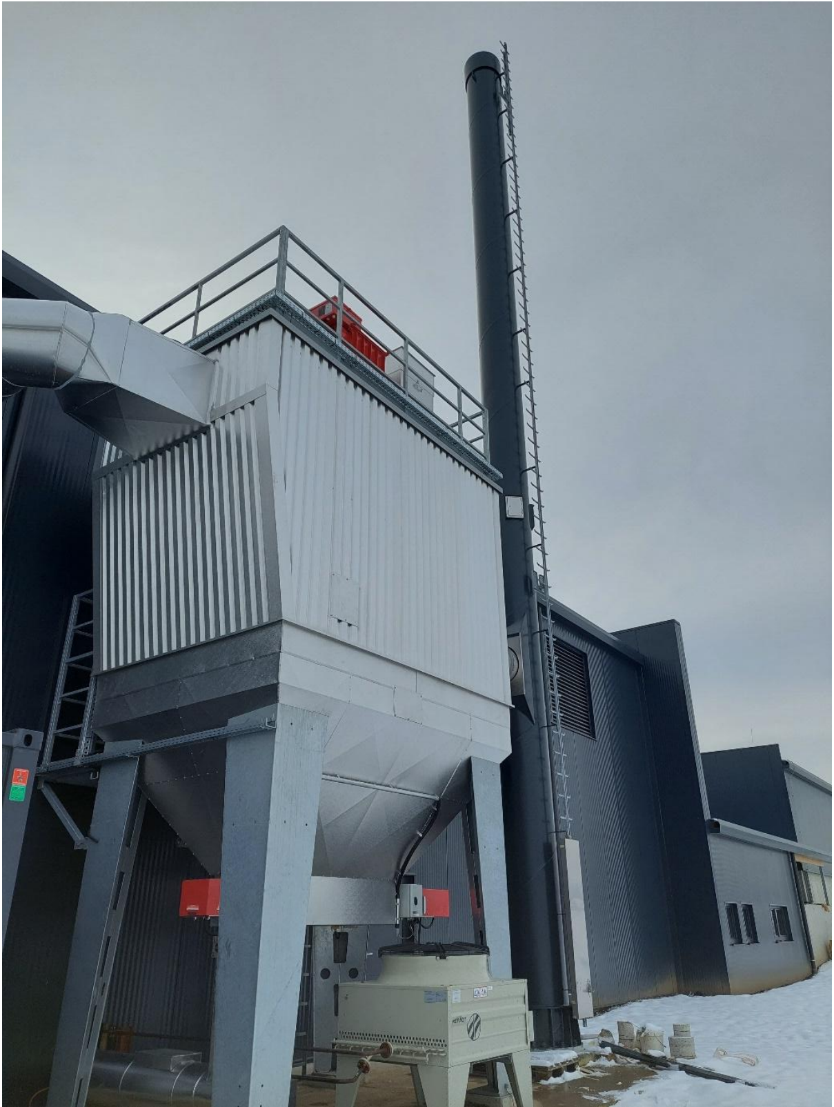
Figure 8: Electrostatic precipitator and chimney (Source: BC Regionalwärme Group)
